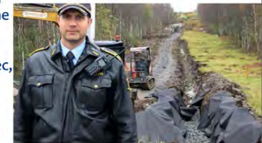
Stein Kristian Hansen is building a ‘friendly, Norwegian’ fence on the Russian border
